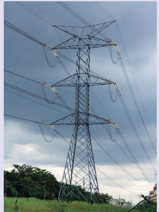
■ Figure D4.17 Transmission lines transfer electrical power around countries
