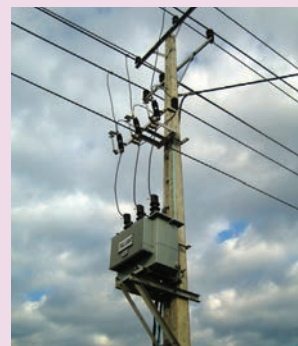
■ Figure D4.15 A transformer on a road-side pole
