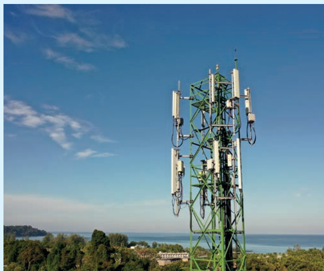
■ Figure C3.9 Typical aerials for transmitting mobile phone signals
